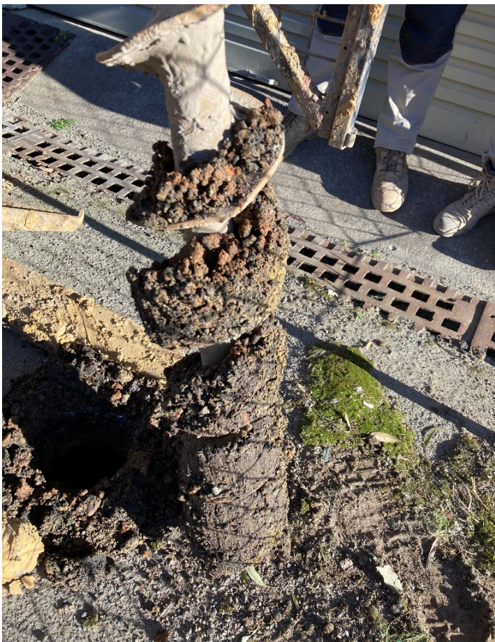
Fill material encountered in BH6a
