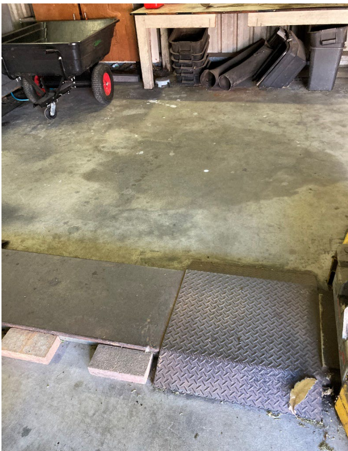
Moderate oil staining on the concrete beneath the hoist of the Yard Maintenance Shed. No cracks or deterioration of the surface was noted
